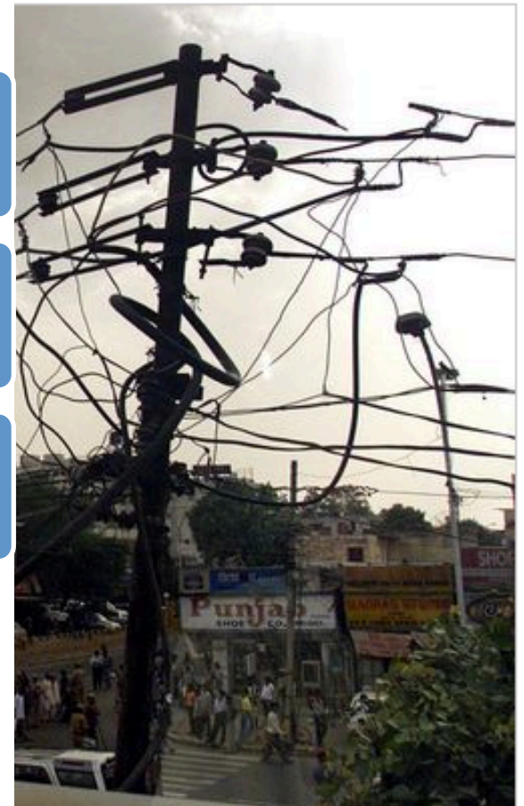
A tangle of wire atop this electricity pole in New Delhi, India in 2002 was testament to the capital city's power theft problems. Since then in North Delhi, automation has helped slash electrical losses.
