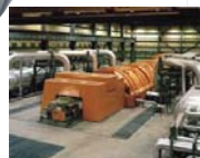
Power generation and distribution
