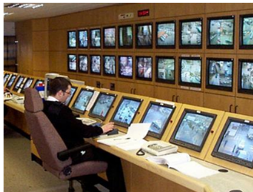
Fig. 1. Typical CCTV control room with video feeds from several cameras
