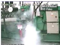
Experimental cyber-attack caused generator to self-destruct.
